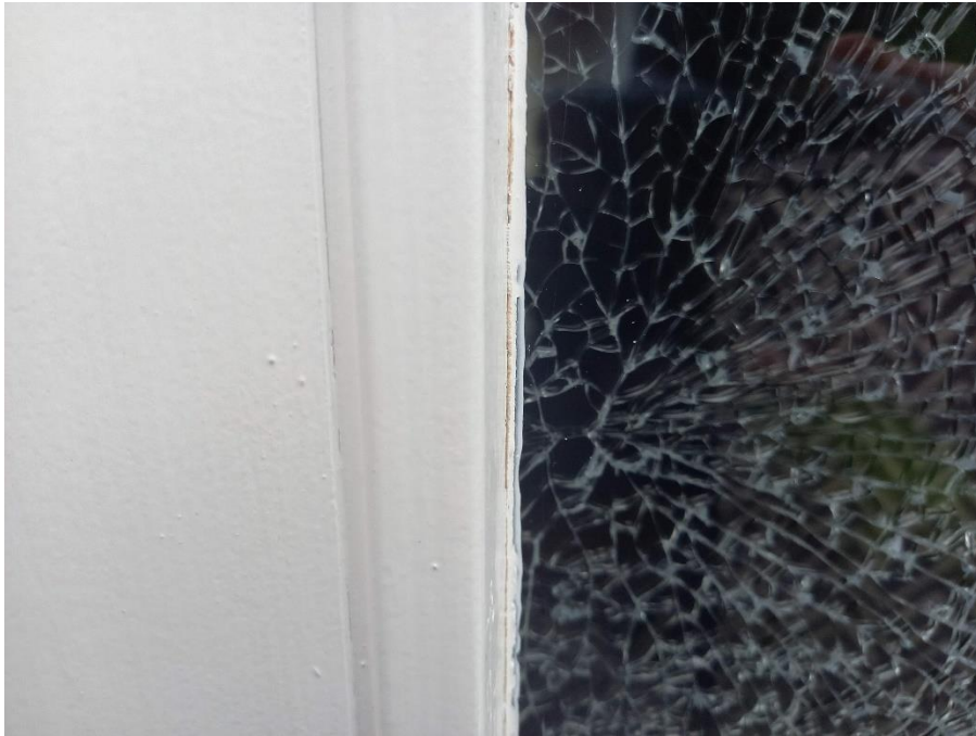
Broken window glazing units due to incorrect fitting and no expansion
